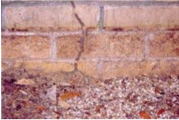
Termite shelter tubes on foundation wall.
